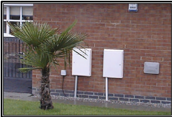
Exposed cables can leave property vulnerable to crime
