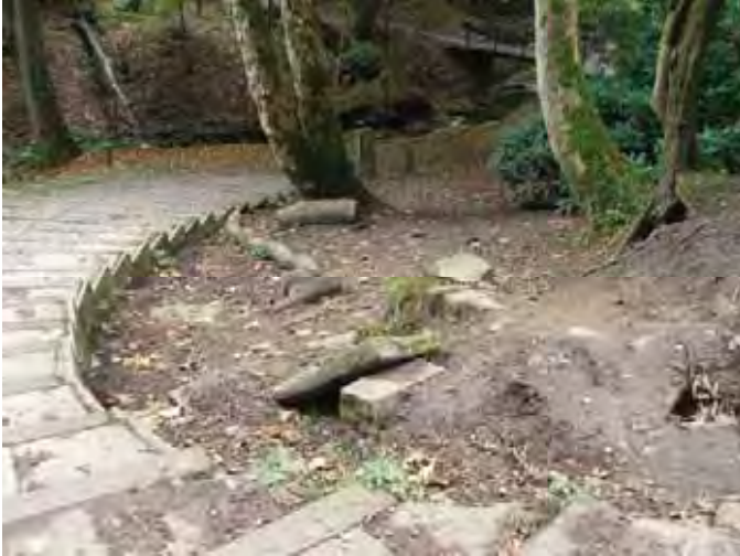
48: Erosion of steps leading down to the main footbridge
