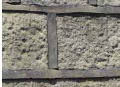
Fig.86: poor quality pointing
