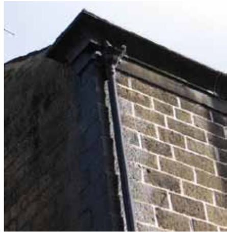
Fig.79 Watershot masonry and stone gutter on Bury New Road
