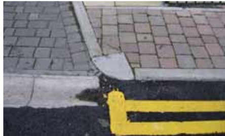
Fig. 56: Recently laid concrete setts and kerbs on Cross Street with obtrusive yellow lining
