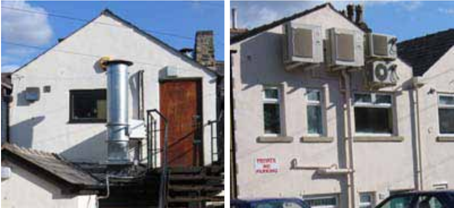
Figs.93 and 94: Examples of visually intrusive air-handling units and flues at the rear of properties on Central Street
