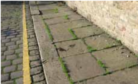
Fig. 55: Sandstone setts and paving on South Street to the rear of Peel Brow
