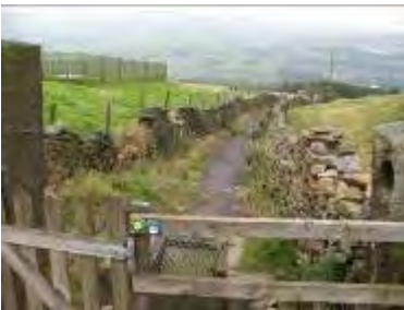
Dry stone Walls in Poor Condition
