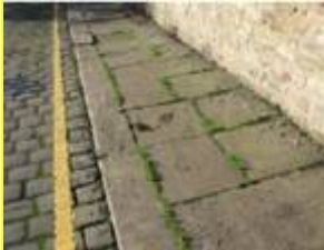
Traditional stone setts contribute to the character of the street scene, but need careful repair
