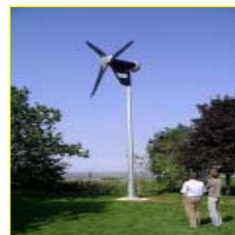
6KW Proven Turbine located within the grounds of a school (Source: TV Energy)
