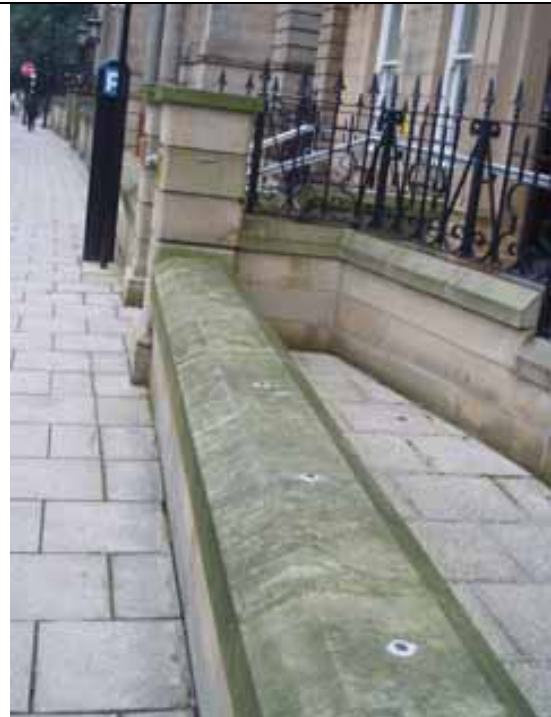
Fig. 51 Railings now missing from Textile Hall
