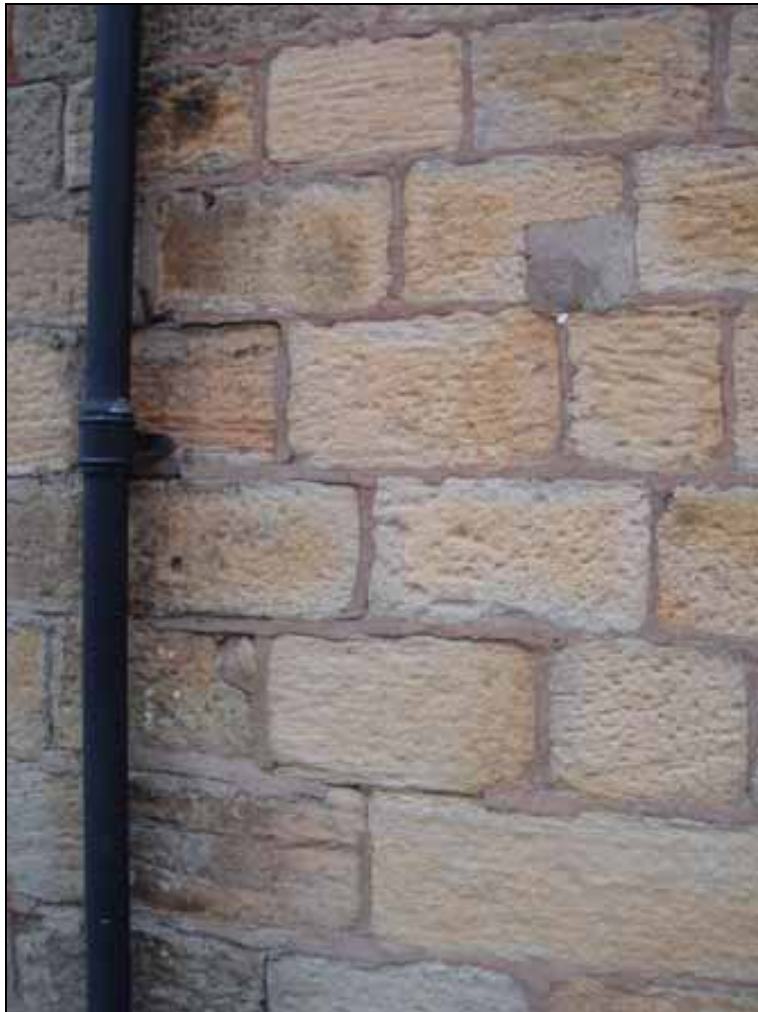
Fig. 99 Poor repointing, rear of St Marie's Church, Manchester Road.
