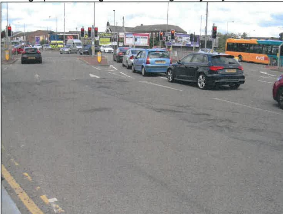
Photograph 2 – Failing Thin Surfacing Derby Way
