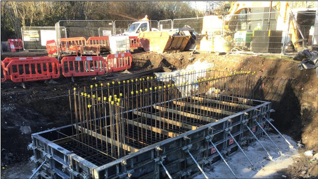
Roch Valley Greenway Crossing under construction – providing a crossing over the river for pedestrians, cyclists and horses.
