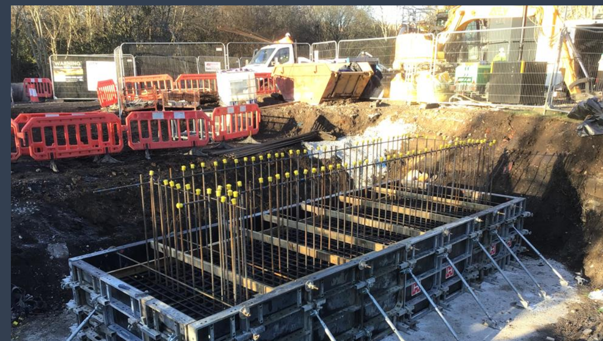
Roch Valley Greenway Crossing under construction – providing a crossing over the river for pedestrians, cyclists and horses.
