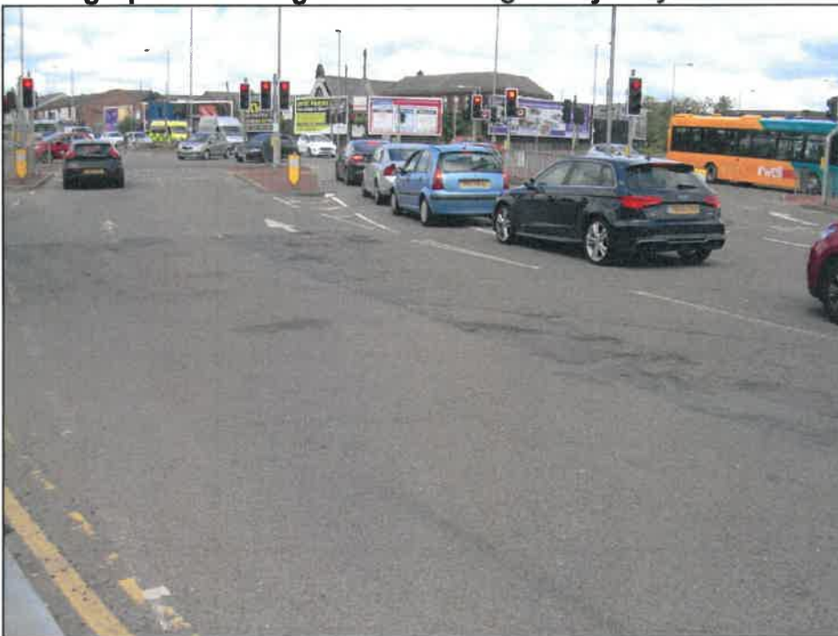
Photograph 2 – Failing Thin Surfacing Derby Way
